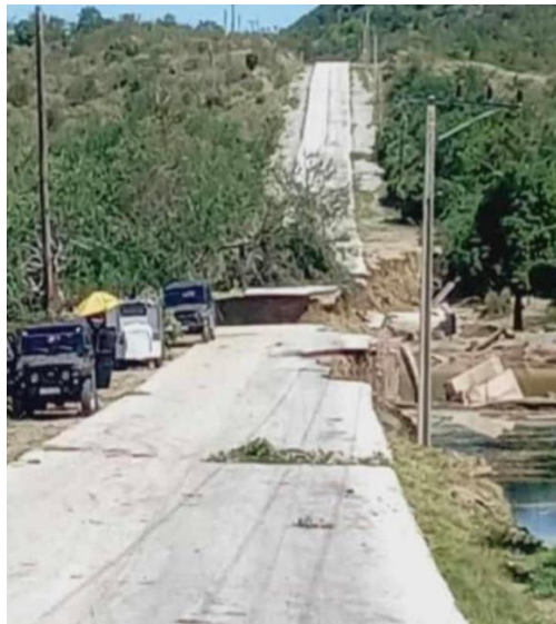
Access road washed out.
