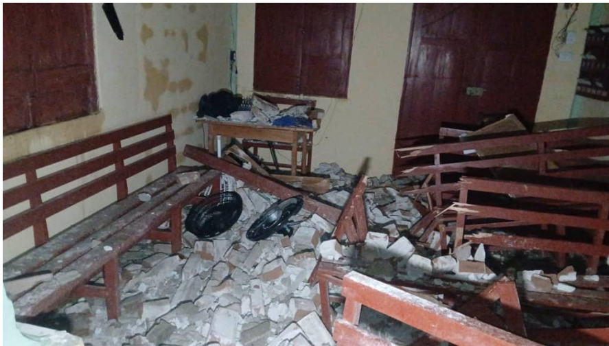
Inside 6 th Baptist Church Baracoa. The roof collapsed.
