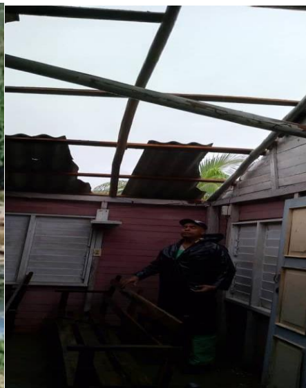
Many metal roof peeled off buildings.
